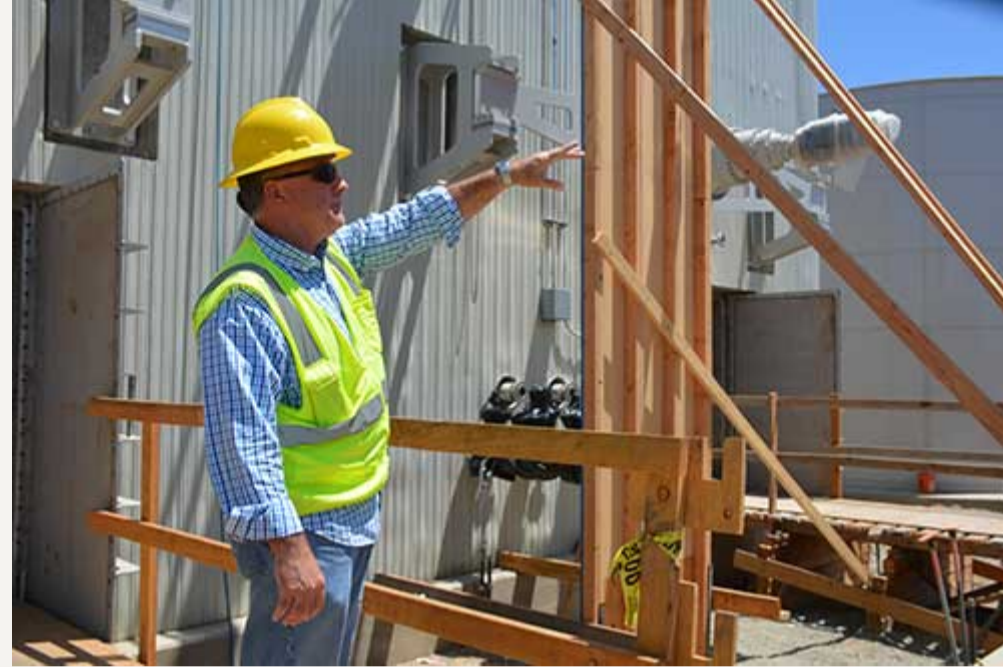
Project Manager Mike Silva inspects construction of the world's largest anaerobic digester in Perris, which will convert hundreds of millions of pounds of organic waste each year into fertilizer and fuel to power heavy-duty trucks.
