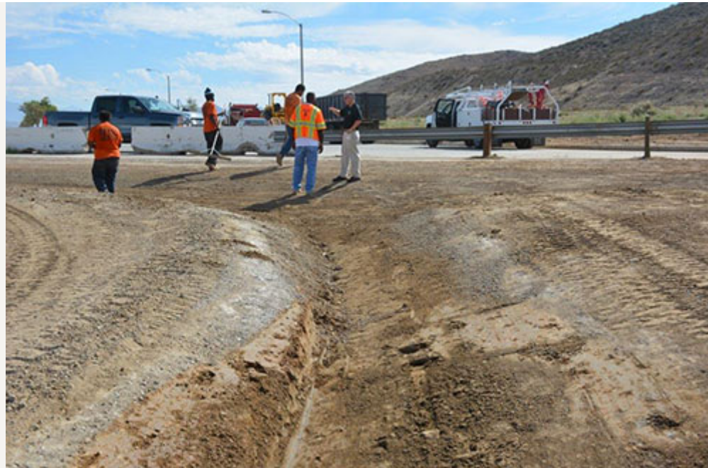
Perris Assistant City Manager Ron Carr (black shirt, right) meets Wednesday with members of a construction crew building a drainage channel to move water away from residences in the Monument Park and Monument Ranch neighborhoods in the City's south end.
