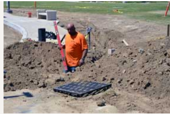
Workers re-grade the turf areas at Monument Ranch, resulting in improvements that will keep grass greener while reducing the likelihood of flooding.
