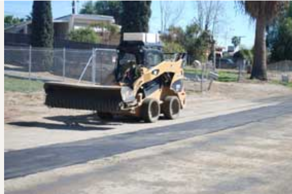
Construction of the sewer system required persistence by the City of Perris and its partners and patience from Enchanted Heights residents. Here, a bulldozer works on a street in 2012.
