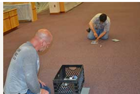
Workers install new electrical outlets and squares of carpeting at the Cesar E. Chavez Public Library in Perris.
