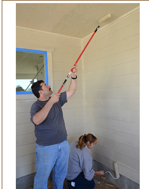
Hugo Gomez and his wife, Laura, paint the exterior walls of their new home, built as a result of a partnership between the City of Perris and Habitat for Humanity.
