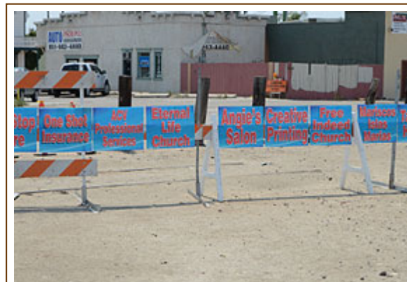
Signs inform people that all D Street businesses remain open during construction.
