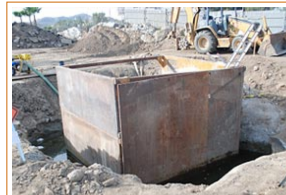
This lift station, under construction in Enchanted Heights, will channel wastewater from the neighborhood as part of the three-year, $15-million sewer project.
