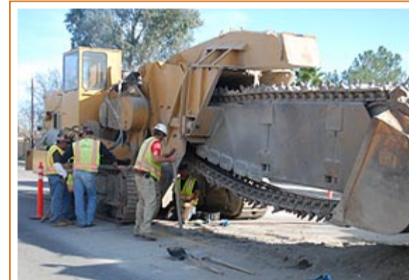
Construction work on the Enchanted Heights sewer system is underway, as trenching machines cut through pavement so sewer mains can be installed.
