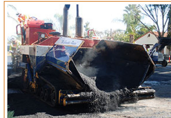
Part of the improvements consisted of installing a new layer of blacktop at the Perris City Hall campus.
