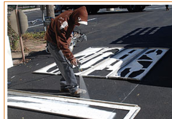
A worker stripes the parking lot as part of the construction improvements.
