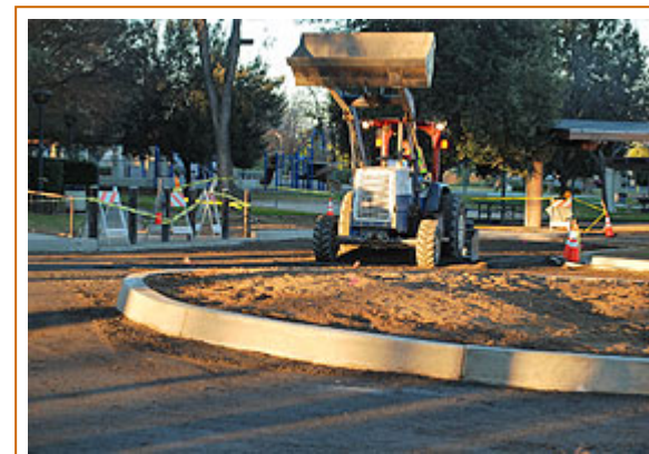
A skip loader cuts a traffic circle at the Perris City Hall Campus, linking three lots into a single parking area.
