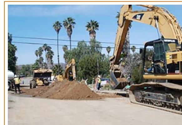
Construction crews have been hard at work installing main line sewers in Enchanted Heights.
