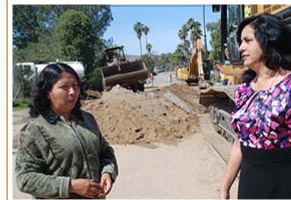
Enchanted Heights resident Yolanda Hernandez (left) discusses the sewer project with Maria Elena Kennedy of the City of Perris.
