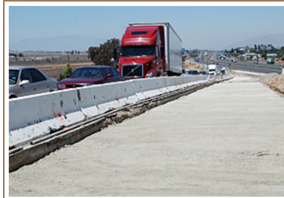
Traffic exiting southbound I-215 often backs up. The addition of another exit lane should help remove a major bottleneck.
