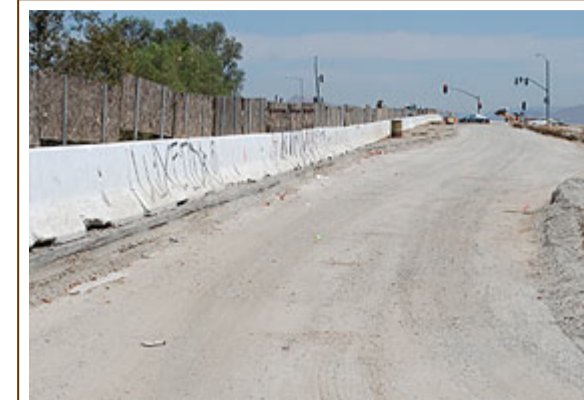
The new expansion of off-ramps at Ramona Expressway and I-215 in Perris includes the addition of another lane for traffic exiting the freeway.
