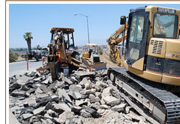
Heavy machinery remove blacktop while making improvements to the on-ramp at I-215 and Ramona Expressway. Work on the $7.5 million project should wrap up by year's end.
