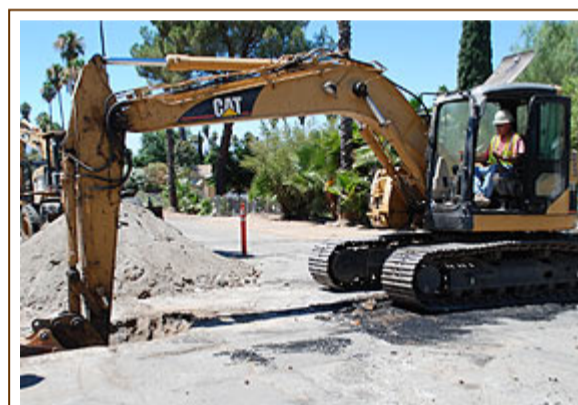
A trenching machine cuts a path for a lateral connection Thursday (July 26) in Enchanted Heights.
