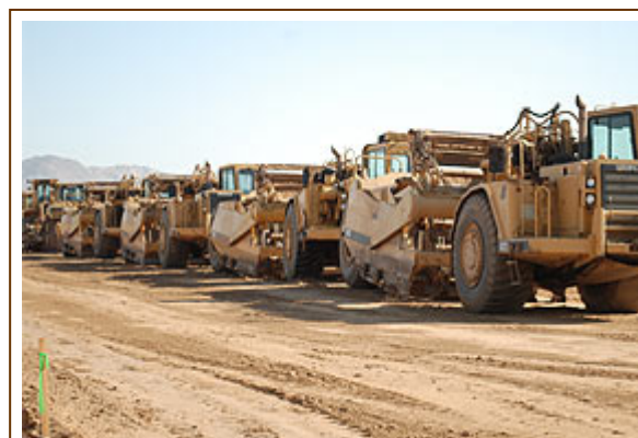
A line of earth-haulers stands ready to transform the vacant field on Trumble Road into a world-class aquatic center.
