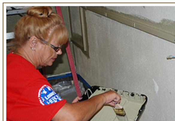
Jolene Oakley paints a wall in the Perris High School culinary kitchen.
