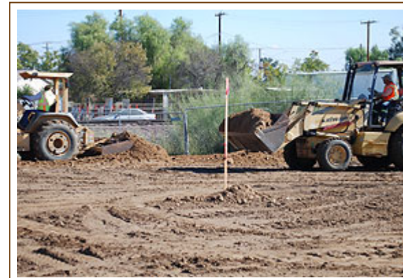
Work on the project began several weeks ago and is expected to be completed in mid-2013.
