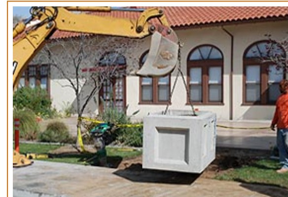
A crane lowers the 3,500-pound vault that will encase the Centennial time capsule into the ground just outside the Perris City Council Chambers.
