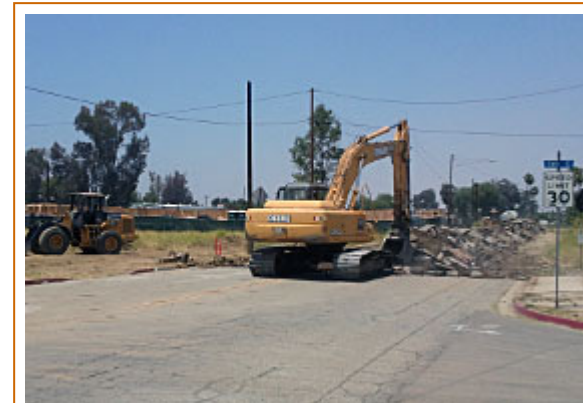
Construction work has closed D Street between Eighth and Tenth streets in Perris.
