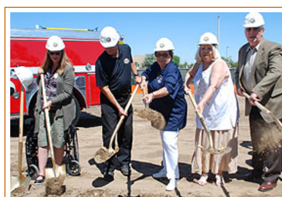
Perris City Clerk Judy Haughey, City Councilman Mark Yarbrough, Mayor Pro-Tem Joanne Evans, City Councilwoman Rita Rogers and Mayor Daryl Busch dig to break ground at the new station.
