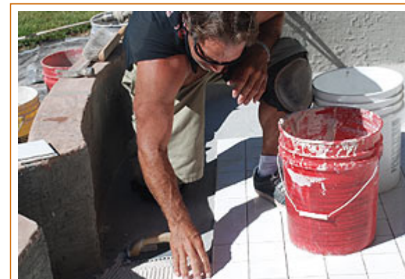
A tile-setter works on the floor of the iconic fountain outside Perris City Hall.
