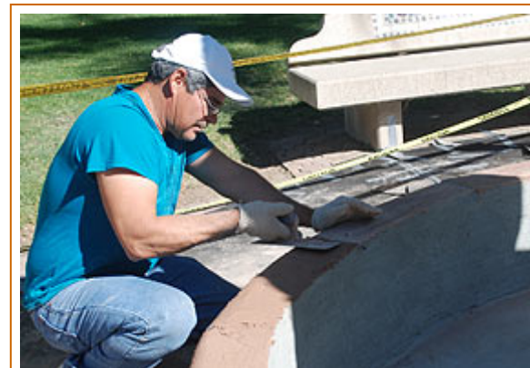
Part of the construction included putting new sealant around the base of the fountain.
