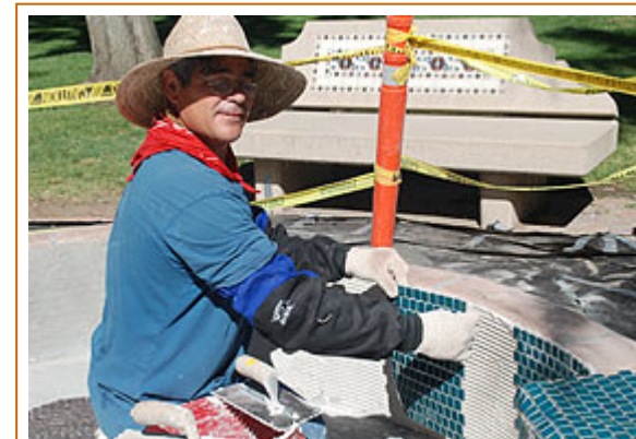
The sides of the Perris City Hall fountain were replaced with new ocean-green tiles.
