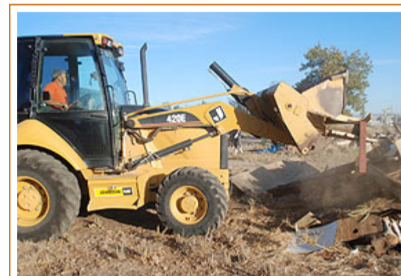
Perris Public Works employee Eddie Gutierrez operates a loader while cleaning up at a residence on Mapes Road near Perris Valley Airport.
