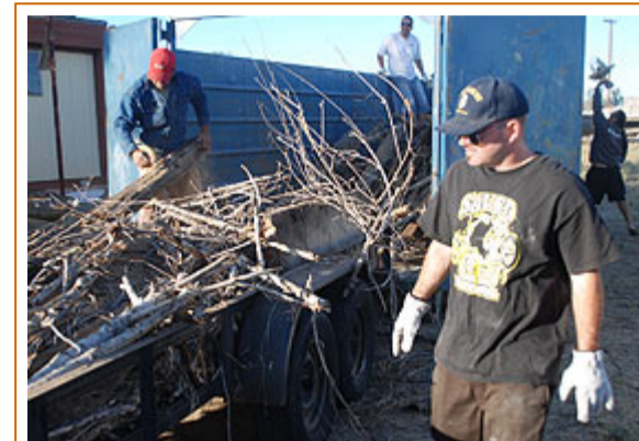
Zac Mullinax helps load a Dumpster while working at a house on East Sixth Street.
