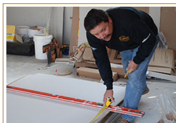
Rene Avila, Assistant Director of Development Services for the City, measures a piece of drywall before cutting it and installing it inside the garage at the Second Street home.
