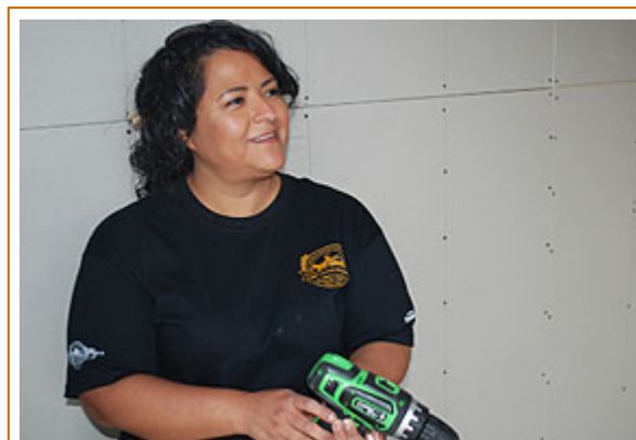
Administrative Services Manager Isabel Carlos gets ready to install drywall Thursday afternoon.
