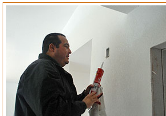
Perris City Manager Richard Belmudez caulks a ceiling at the Habitat for Humanity house.
