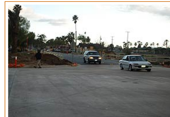
Traffic moves north on D Street from First Street to San Jacinto Avenue late Tuesday afternoon. The thoroughfare reopened to vehicles after about three months but construction continues on other improvements along D Street.
