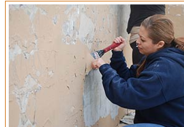
Angie Soria removes peeled and crack paint from the handball court at Paragon Park.
