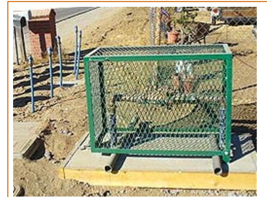
Typical backflow device.
