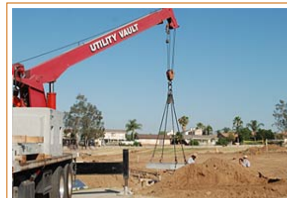
A crane lowers part of the foundation for a new gym into place.
