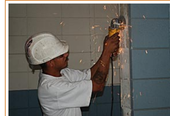
Sparks fly as Michael Navarro grinds a piece of metal off a doorway at the former Perris Police Department complex, which is being converted into an auto-repair and body shop.
