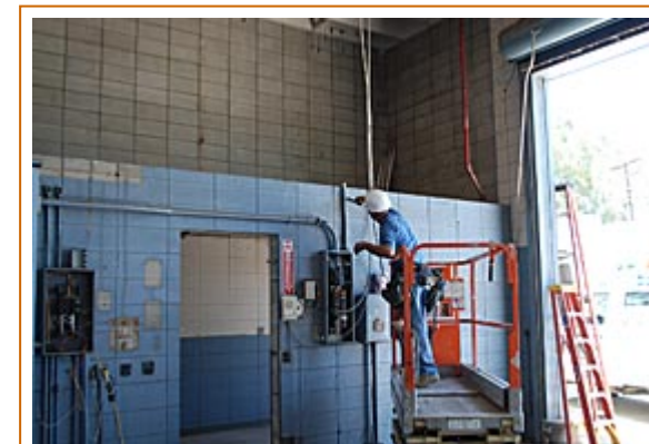
A worker rips off electrical conduit as part of the ongoing renovations.
