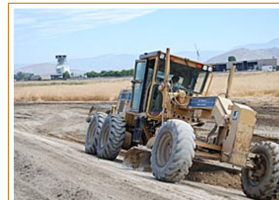
A road-grader gouges out dirt to make a new drainage ditch to help end flooding at Mapes and Goetz roads. The Perris Valley Airport wind tunnel is in the background.
