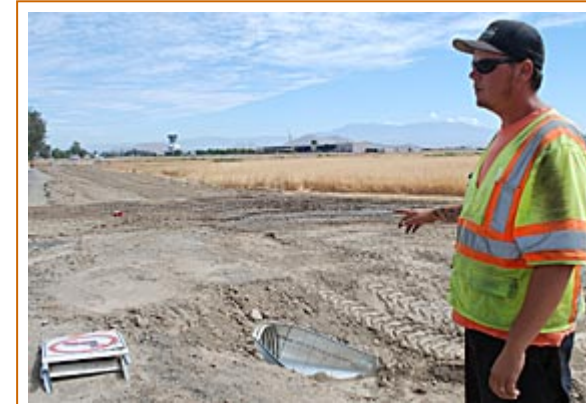
Construction foreman Doug Nace points to a 36-inch drainage pipe that will carry water from the intersection to the San Jacinto River channel.
