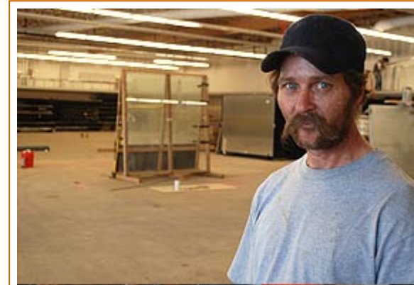
Construction foreman James Taylor inside the Rio Ranch Market on 4th Street, where a construction crew is working to get the store open by December.
