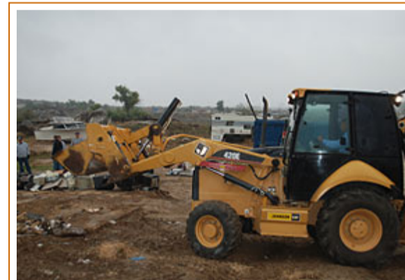
Public Works employee Juan Lemus operates a loader at a residence in the City's west end.
