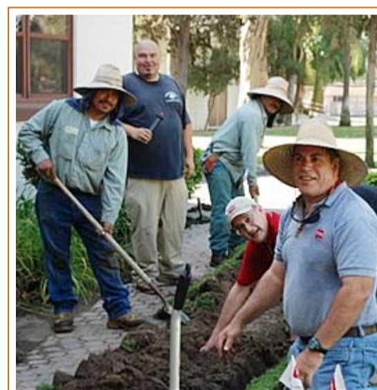
Workers dig a trench to install new irrigation equipment at the Perris City Hall Campus.
