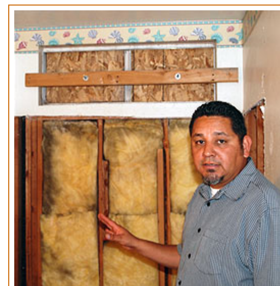
Perris housing consultant Anthony Perez examines construction rehabilitation progress at a residence on Red Bud Place. City contractors were quizzed by interested residents even before the work was finished.
