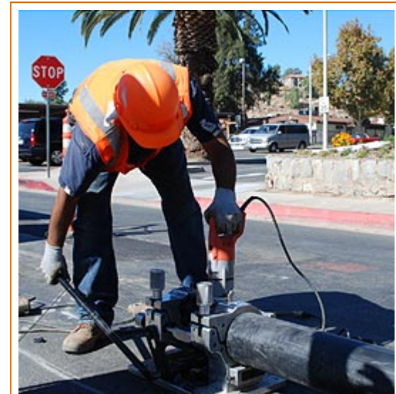
A worker readies the machine that will snake new flexible piping inside an existing concrete pipe near Perris City Hall.
