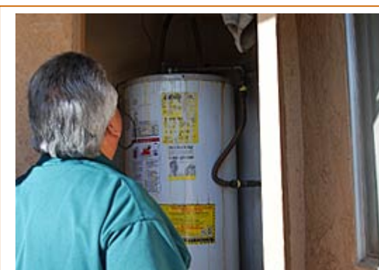
Gomez checks out a broken water heater.
