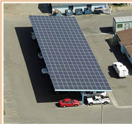
Aerial views of Perris solar-panel carports which were honored this week at the League of California Cities.
