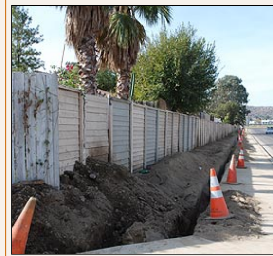
A new perimeter fence and landscaping is going in along Perris Boulevard in the Rancho Las Perris neighborhood.
