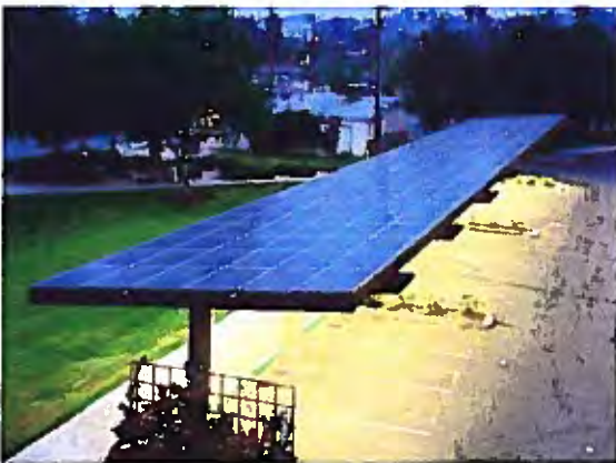
Perris Civic Center Solar Carports
