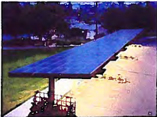
Perris Civic Center Solar Carports
