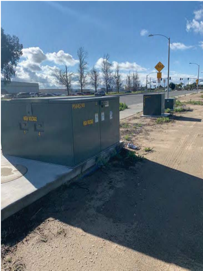
Transformers Along the Eastern Border
