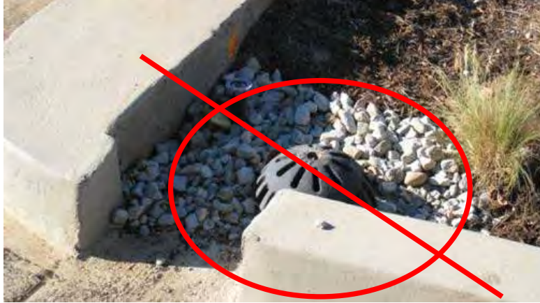
Figure 6: Incorrect Placement of an Overflow Inlet.
