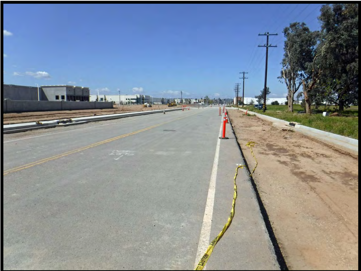
Overview of Markham Street Frontage at Project Site, towards Perris Blvd., Perris (W)
