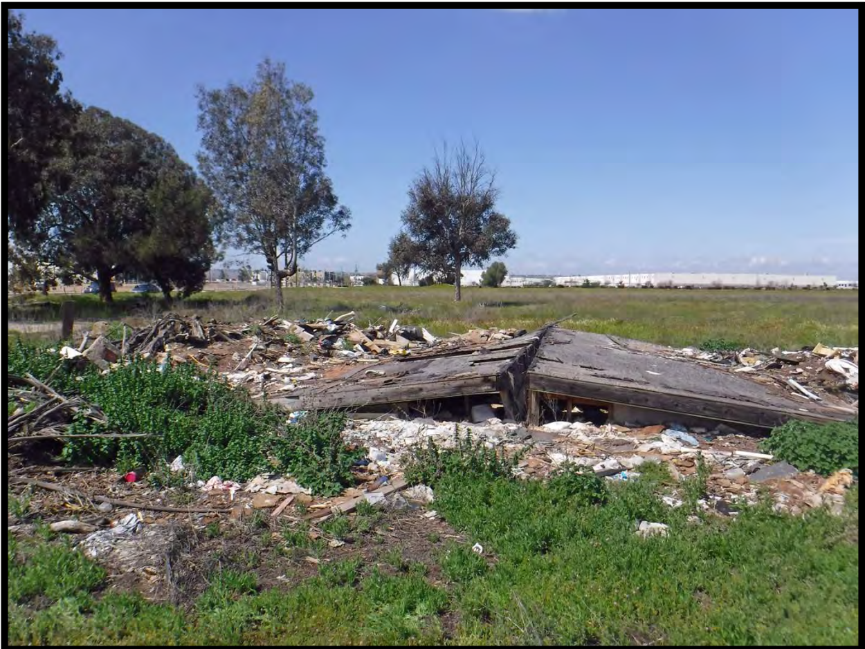
Collapses Roof Identified near Markham Street, Parcel -031, Perris (W)
