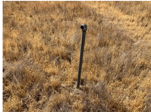
16. Domestic water supply at Parcel 7
