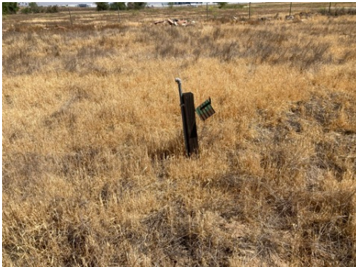
15. Domestic water supply at Parcel 6
