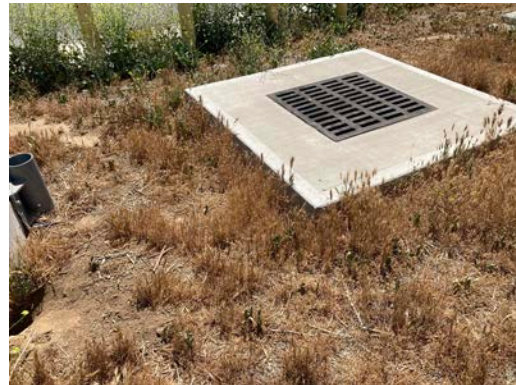
22. Stormwater pump system to northeast of Parcel 1
