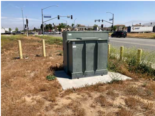
21. Pad-mounted electrical transformer to northeast of Parcel 1
