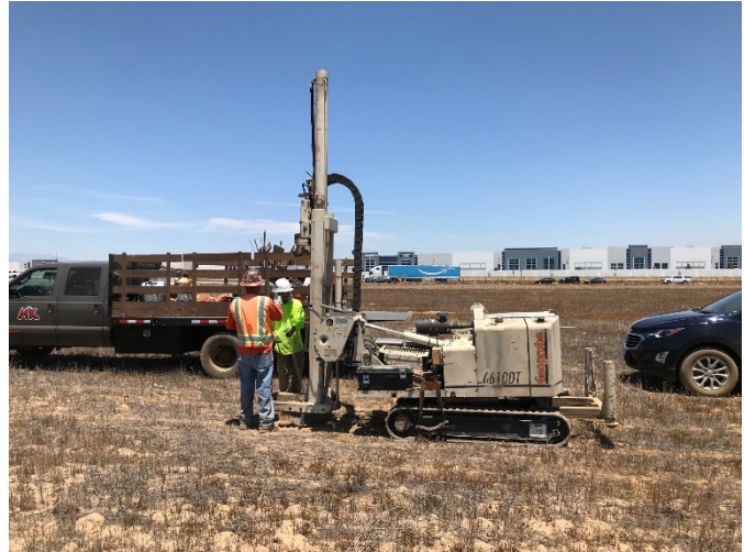
8. Geoprobe direct-push drilling rig set up at soil boring SB-6 in the northwestern portion of the Site
