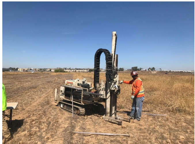
4. Geoprobe direct-push drilling rig set up at soil boring SB-2 in the east-central portion of the Site
