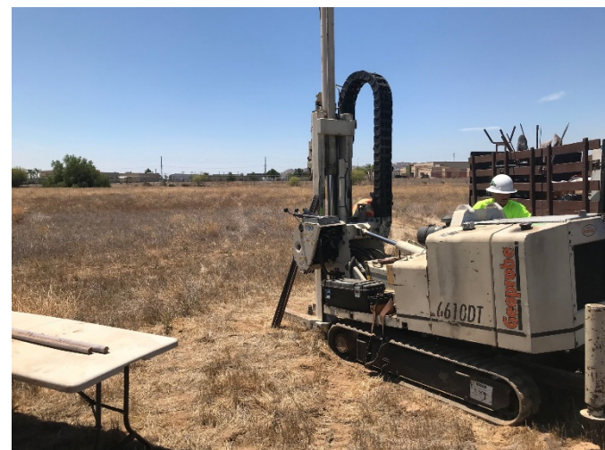
6. Geoprobe direct-push drilling rig set up at soil boring SB-4 in the southeastern portion of the Site
