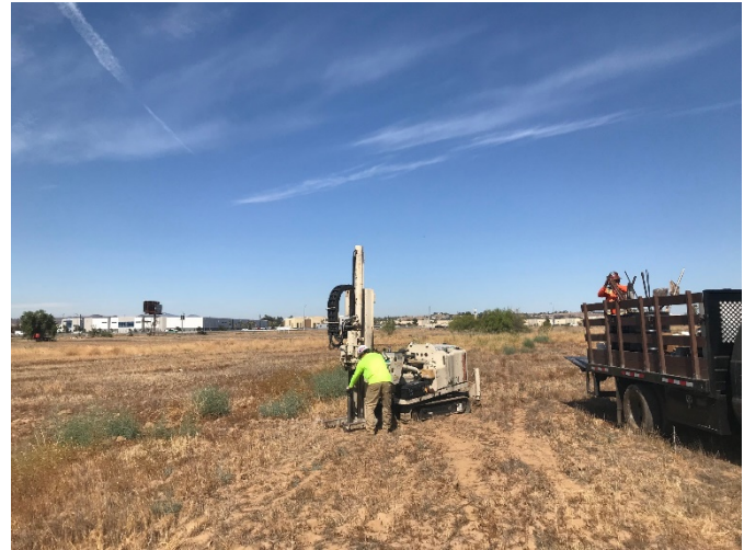
2. Geoprobe direct-push drilling rig set up at soil boring SB-1 in the west-central portion of the Site
