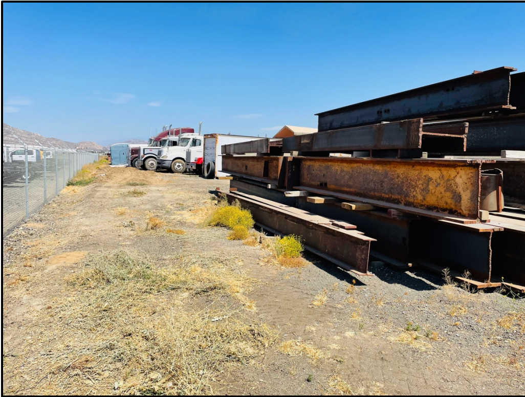
Plate 3: View of parked trucks and stored construction materials on the south side of the project alignment.
