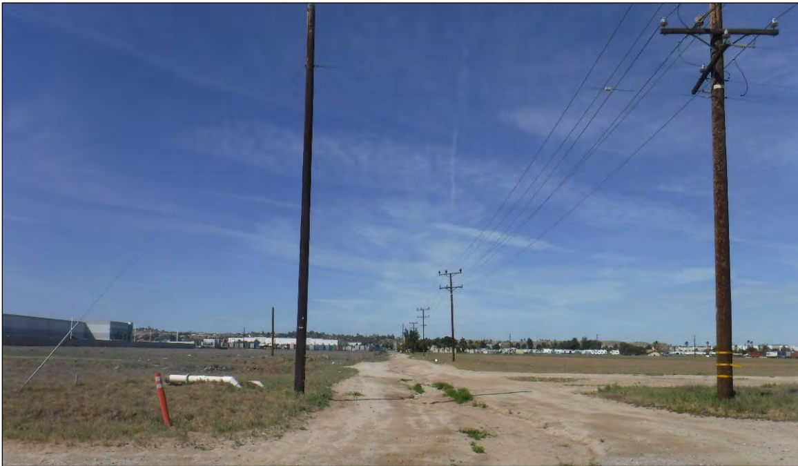
Figure 5-11 Overview of wood pole alignment for West Nance Street Distribution Line, looking west down Nance Street from near the intersection of Nevada Avenue.
