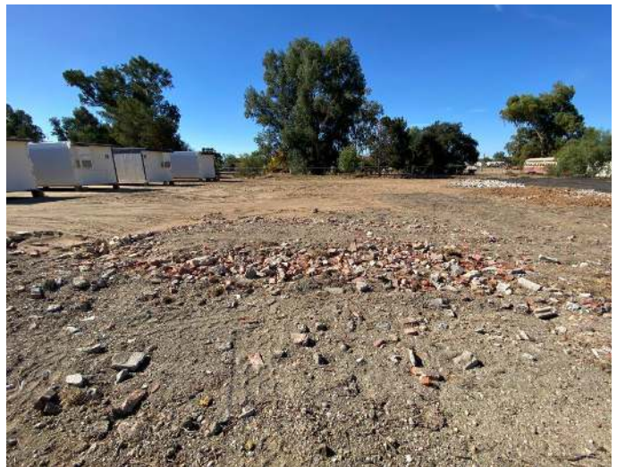
12. View of an area of imported brick, concrete, and stone observed in the central/eastern portion of the Site (presumably used as road-base), looking to the west.
