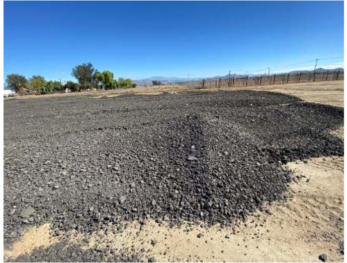
14. View of a typical area of imported asphalt-based placed in the northern and central portions of the Site, looking to the east.
