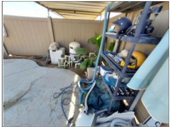
4. Pool equipment at residence at 945 Markham.
