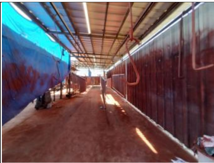
9. HVLP spray paint area 945 Markham.
