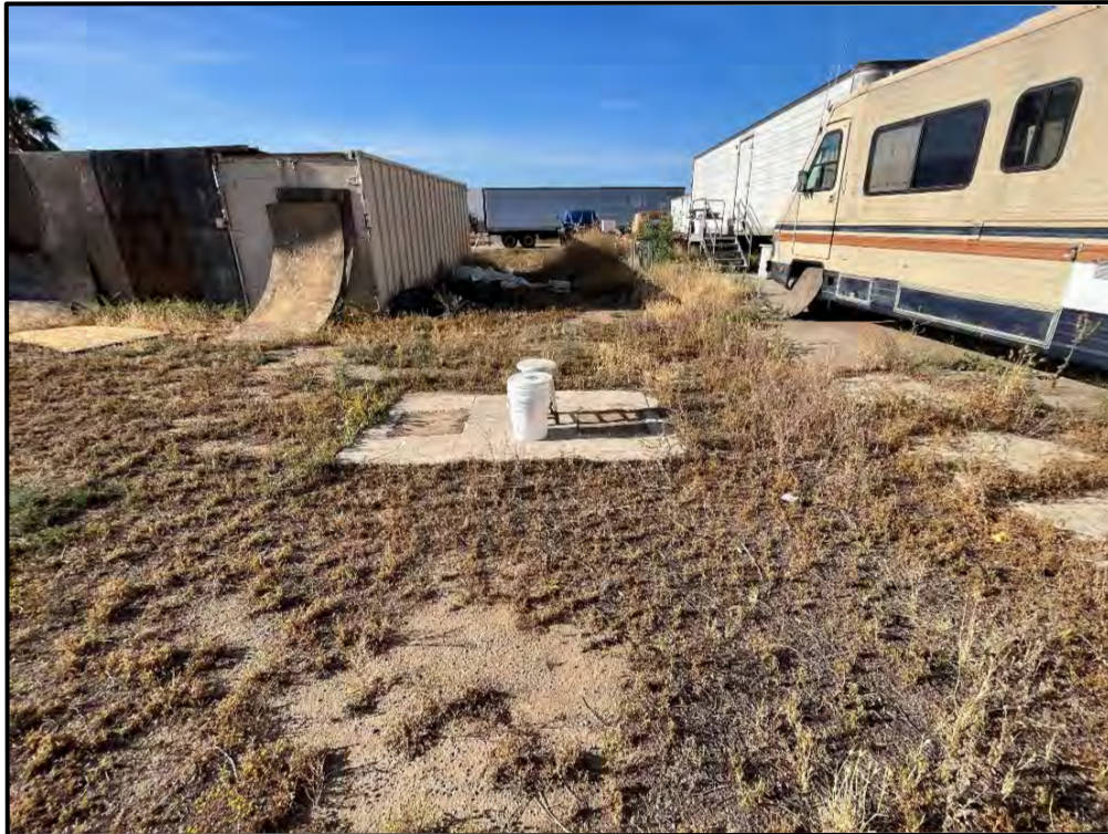
Plate 11: Overview of septic system, facing south.
