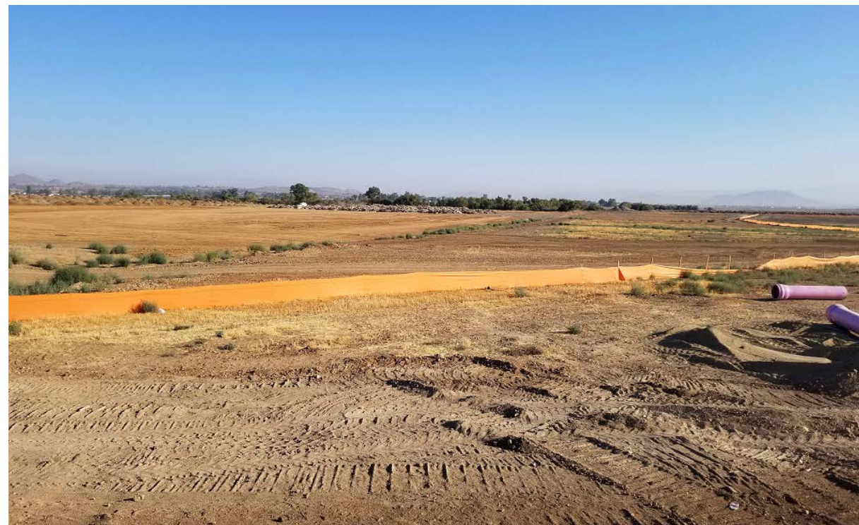
Photograph 4: Representative photo of disturbed portions throughout the Project site.
