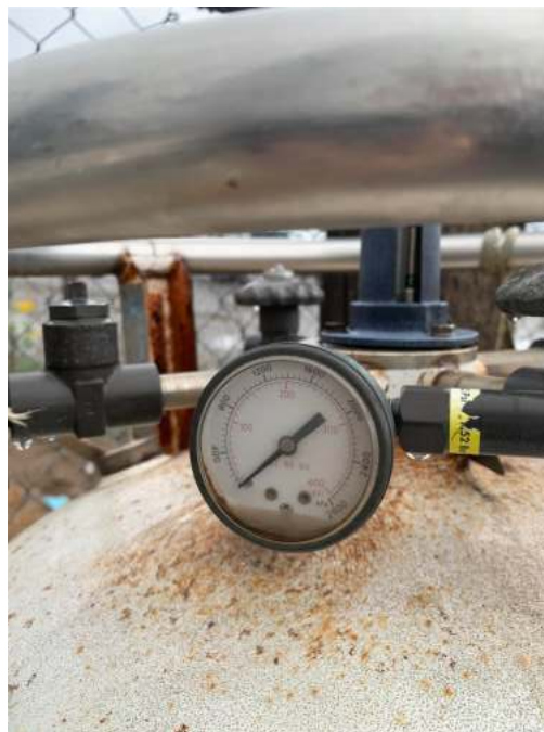
Photo #18 Pressure gauge on nitrogen storage tanks, located in southern portion of the Property. All tank pressure gauges indicated no pressure.
