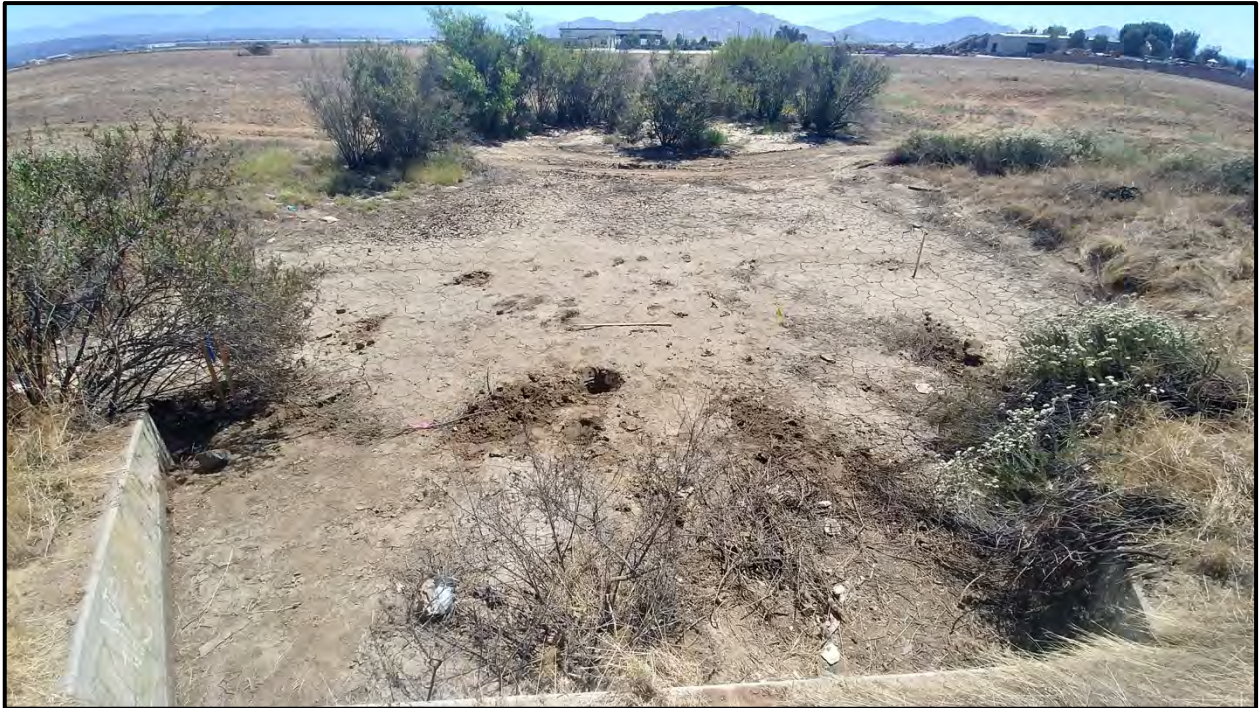
Plate 2: Overview of the modified drainage alignment within the project, facing east from the culvert located at Interstate 215.
