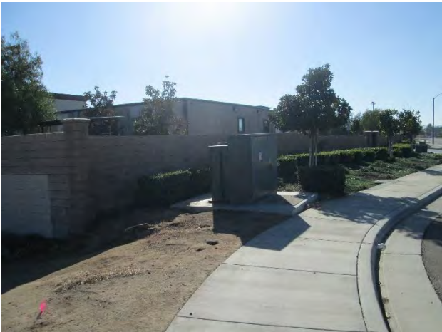
10. Electrical transformer adjoining the southwest corner of the Site.
